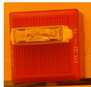
Figure 2 Solvent Fume Hood Fire Alarm Light & Horn Combination
