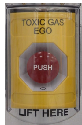
Figure 6 Emergency Gas Off (EGO) Push-Button
