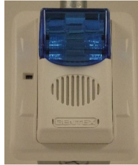
Figure 3 TGMS Alarm Light & Horn Combination
