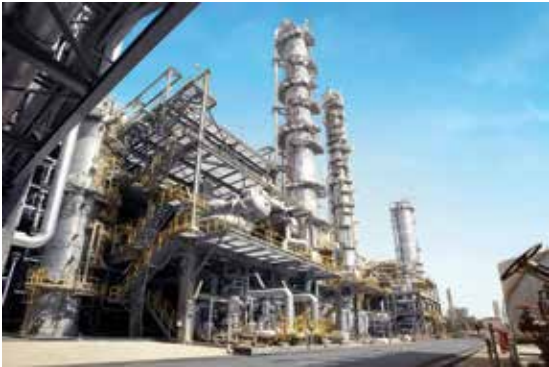
A cumene production plant.
