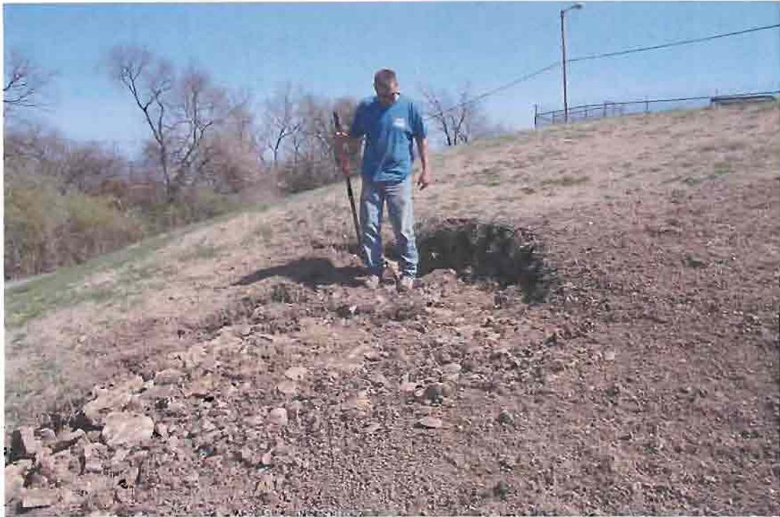
Photo 3: The fill encountered in Test Pit TP-1 was loose and when placed back into the excavation in compacted layers, left this drop off due to not having enough material to level the ground at the test-pit. The drop off was about 1.5 ft tall on the uphill side.
