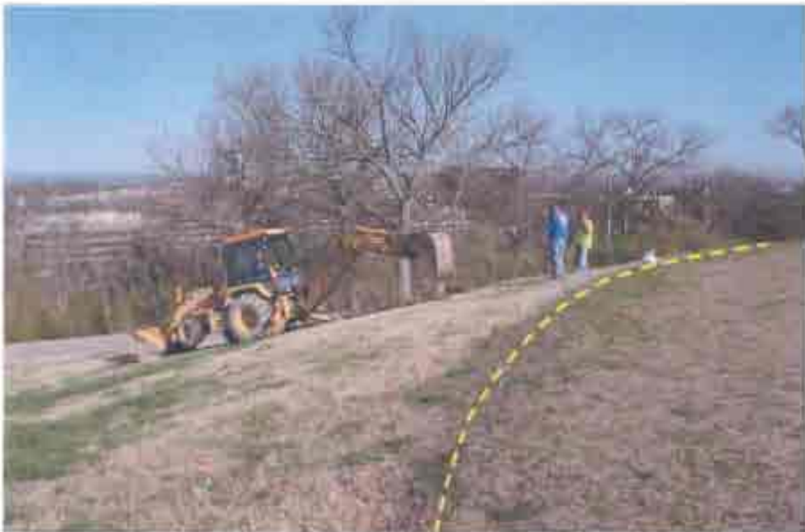
Photo 2: This photo shows the backhoe opening Test Pit TP-1. The dashed line shows the approximate location of the edge of the below ground tank. Per the 1925 plans, about 18 inches of soil caps the tank top. The fill slope is about 3:1 to 4:1 (H:V).
